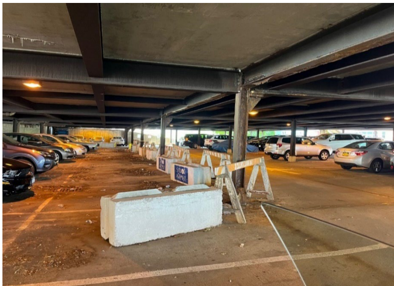
Figure 5 - Flood Damage and Deferred Maintenance at Hunter Tier Lot
